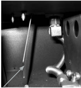
Air shutter rod - located to the left of the valve assembly.
