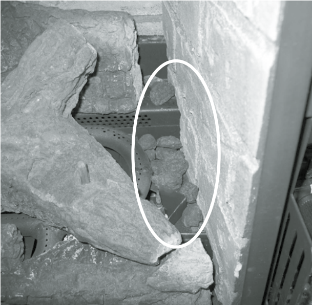
Right side of Burner
