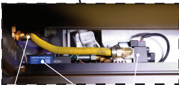
Gas Line Receiver Control Valve
