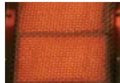
Infrared Bottom Burners (605 & 730)
