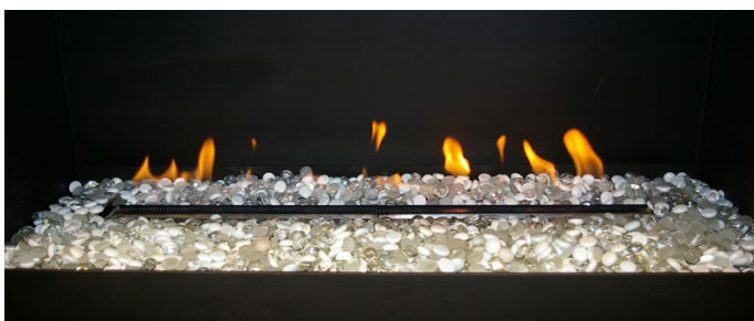
Figure 28a. Operating gas fireplace with firestones surrounding burner tray.
