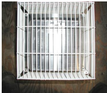
VIEW OF SAFETY CAGE
